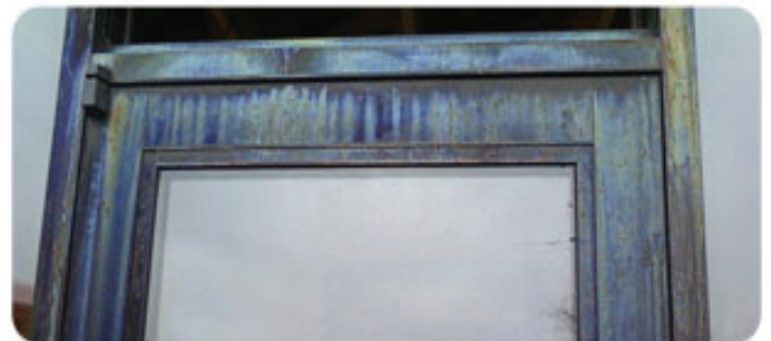
Chemical attack to an anodized finished door
