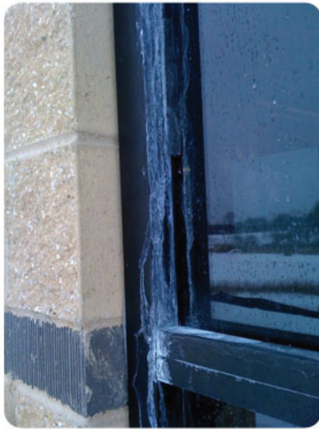
Damage caused to anodized window from brick wash cleaning agent
